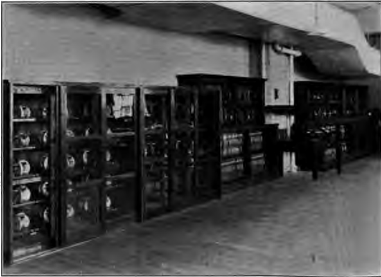
FIG. 118.—Picture of cabinets containing artificial lines.
